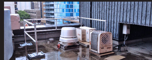
02 GARGOYLE HATCH GUARDRAIL
